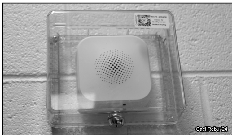
One of the many Indoor Air Quality Sensors present around Sherwood.
